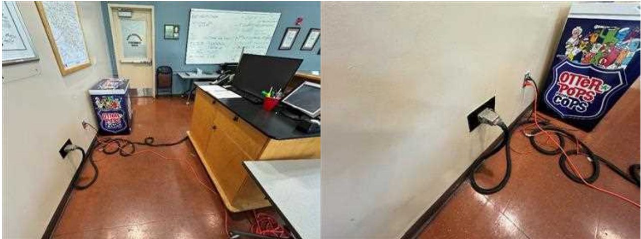
Original equipment was installed with a proprietary custom-made cable that connected to a server room with the control computers and switches. This will have to be replaced and is no longer usable.
