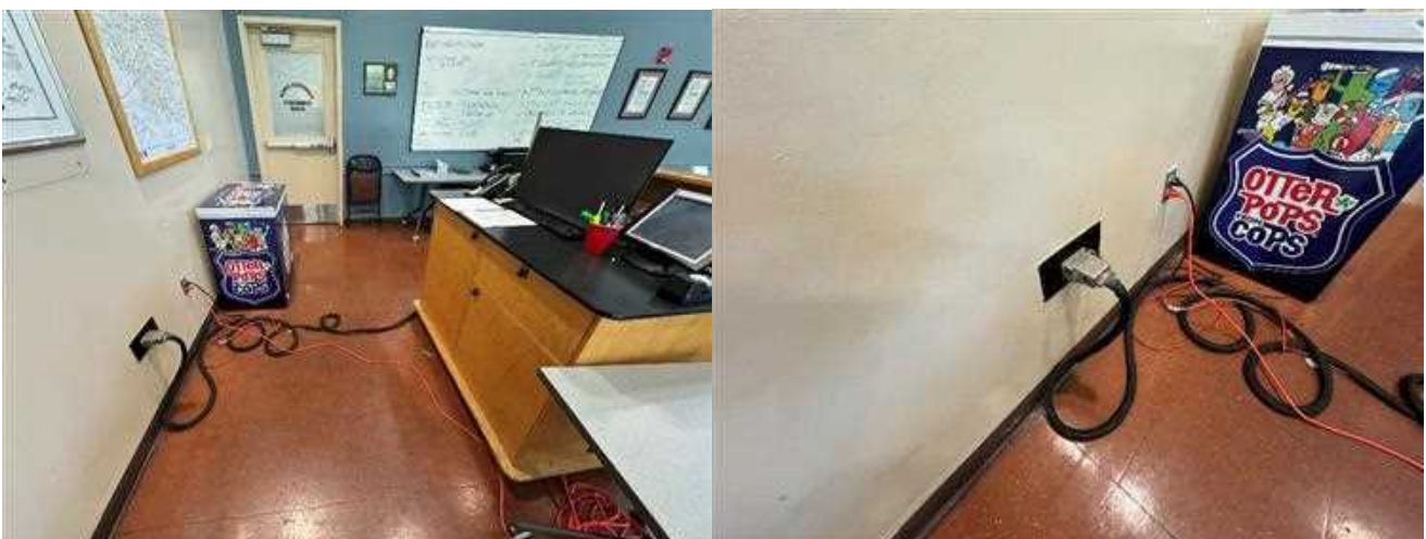
Original equipment was installed with a proprietary custom-made cable that connected to a server room with the control computers and switches. This will have to be replaced and is no longer usable.
