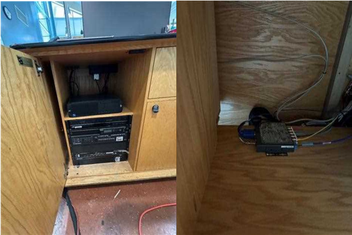
(Left) Equipment inside the podium for switching between various A/V sources. (Right) RCA cables that connect the projector to the podium. These cables will have to be replaced with updated HDMI cables.
