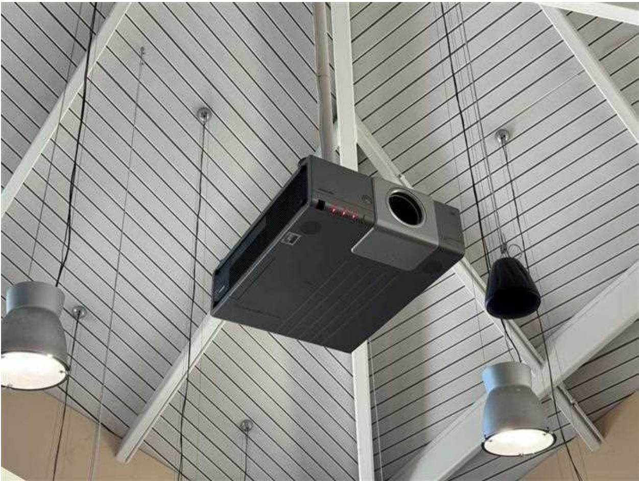
Overhead projector. The project bulbs are no longer available, and it can no longer be controlled. The black cone shaped speaker is also visible. There are six speakers hanging from the ceiling in the room.
