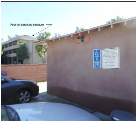
⑤ Exterior mounted wall light shielded from neighboring residential.
