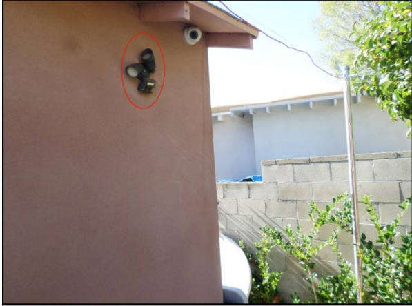
② Exterior mounted wall light pointed away from neighboring residential.
