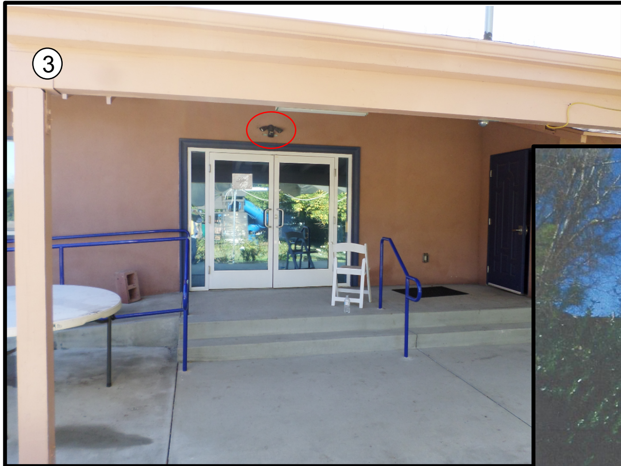
Exterior mounted wall light shielded from neighboring residential.
